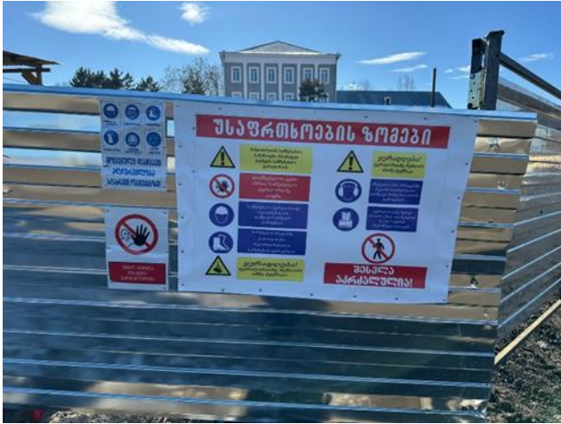
Photo 1 warning signs and banners
